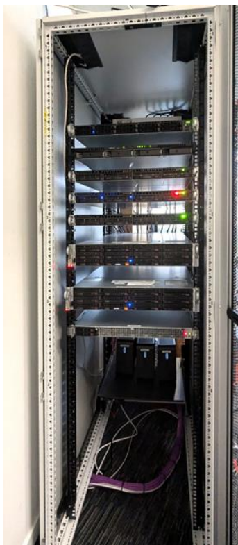
Figure 19: Servers hosting the 6GXR main cluster
